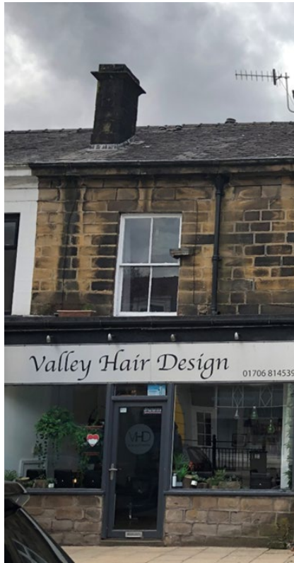
77 Burnley Road. This is the fifth in the row of shops. The original shop front has been replaced.
