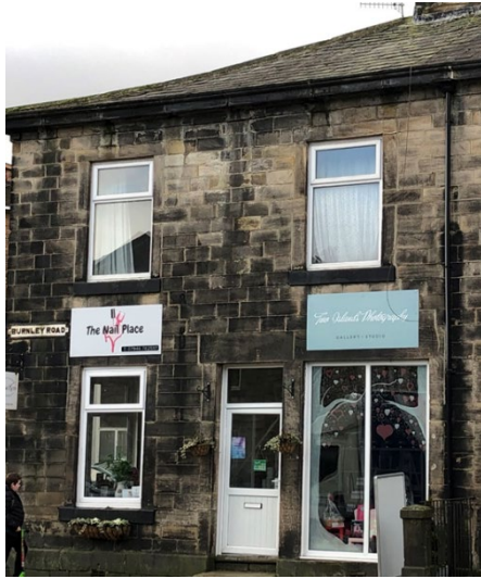
65 Burnley Road. The first of terraced row of old stone-built shops. The original size of shop window can still be seen.
