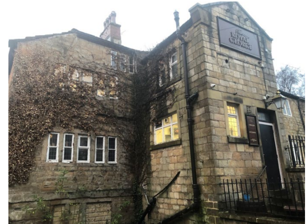
View of the back of the Royal George showing the original level of the road
