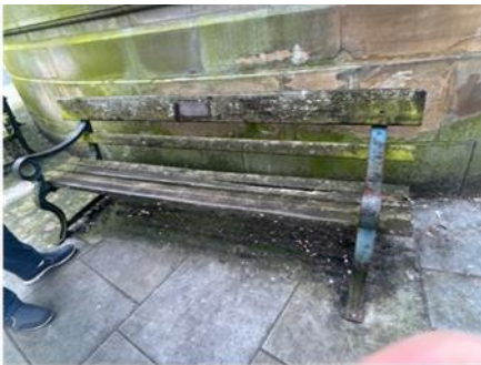
12. The Town Hall - Green mould on the round end of the Town Hall
