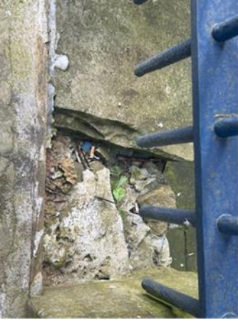
8. The Town Hall - The large amount of bird droppings around the entrance opposite One Stop.
