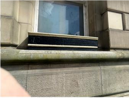
11. The Town Hall - Dirty window frames.
